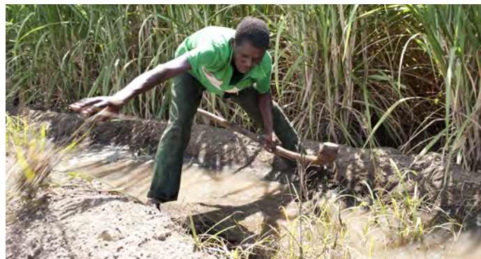
Kasinthula sugar farmer working on the irrigation system
